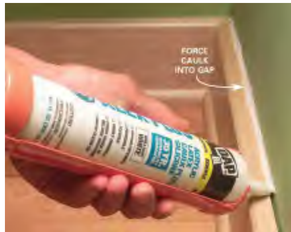
Source: Image by The Family Handyman, "How to Install Baseboard Molding, Even on Crooked Walls," accessed January 24, 2011, http://www.familyhandyman.com/DIY-Projects/Trim/Trim-Carpentry/how-to-install-baseboard-molding-even-on-crooked-walls/Step-By-Step .
